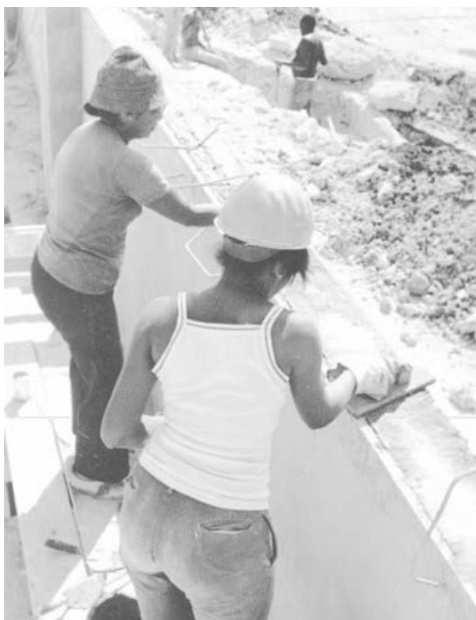
Federation of Cuban Women Cuban women in construction minibrigade in 1988, part of rectification process, as workers from workplaces and communities took part in voluntary labor. They built 100 child care centers in Havana in two years instead of a bureaucratic plan for less than one year. Rectification ended as tighter U.S. embargo exacerbated shortages.
