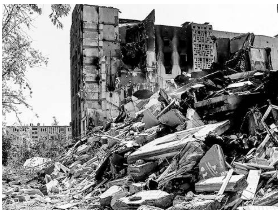
Apartment buildings hit by Moscow's bombardment in Vuhledar, Donetsk region of Ukraine. After most residents of the mining town, which has been fought over for much of the war, were evacuated, Ukrainian forces retreated Oct. 1. Russian troops have suffered heavy losses there.
