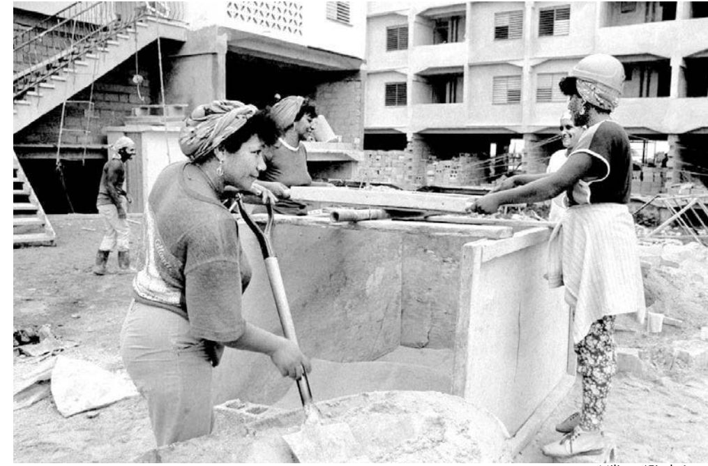
Volunteer minibrigade builds apartment complex in Havana in February 1990. Over 30,000 workers joined construction minibrigades after Fidel Castro launched Rectification Process in 1986. Castro said this effort drew on revolutionary working-class action and example of Che Guevara.
