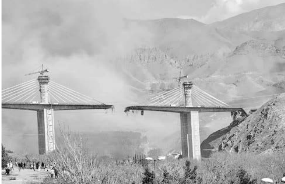
Bridge under construction to link Tehran and Karaj, Iran, was heavily damaged in U.S. airstrike April 2. Washington threatened to destroy Iranian infrastructure, electric grid and bridges.
